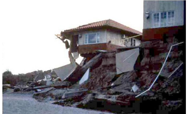
Flood damage, Rillito Creek 1983
